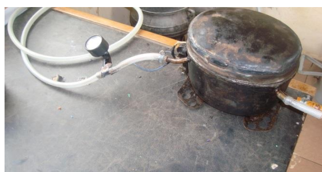
Plate 7: Reciprocating Compressor with Pressure Gauge
